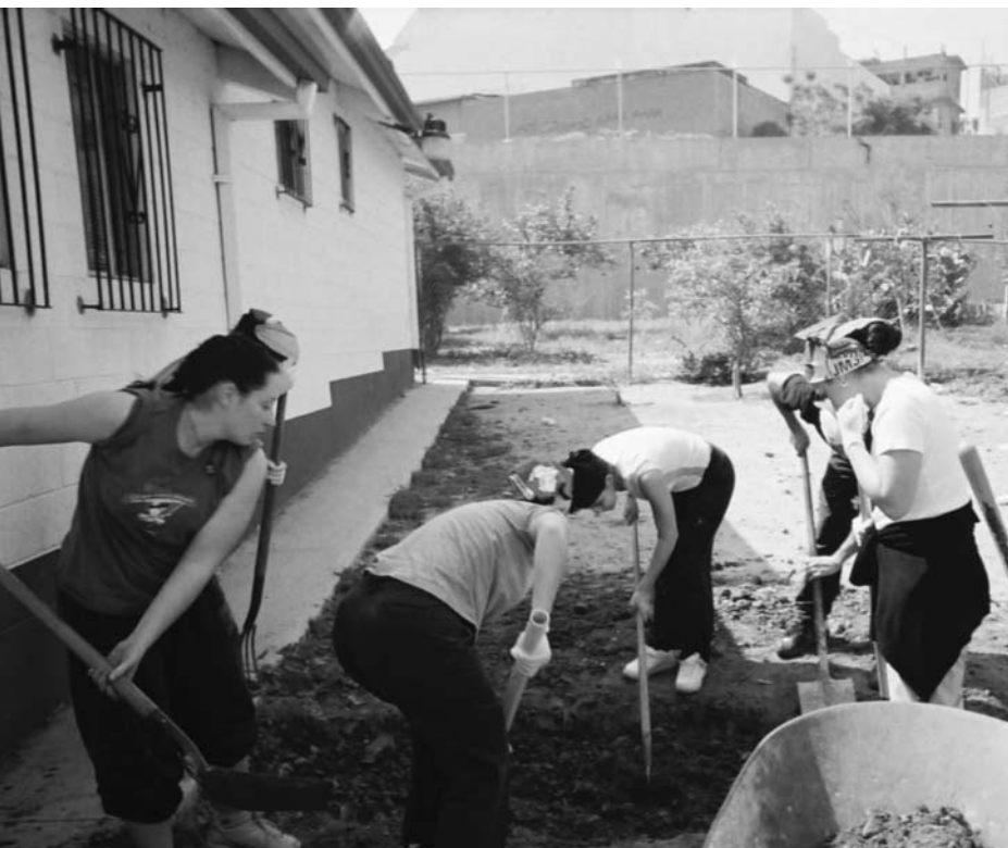
Group breaking the ground to prepare a playground for the Sisters of Charity orphanage in Tijuana.
